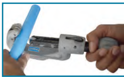
Step 1: Cutting the Tubes
